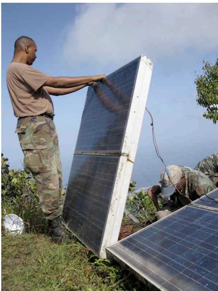
Holding up the solar panels used to power the repeater so that work can get started.
